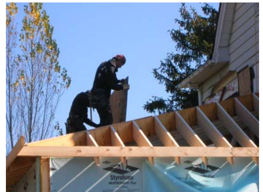
Picture 8: The crew inserting the sheathing panel into the H-clip as they lower it to the rafters.
