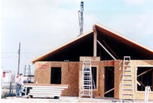
Figure 5 - Roof panels at PATH field evaluation in Texas
